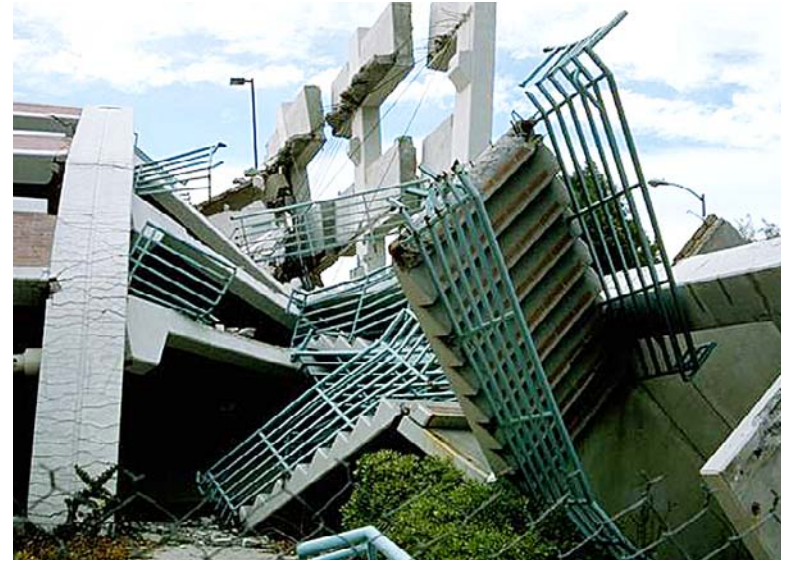
An earthquake destroyed this building.
